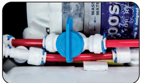
Rinse valve closed, pre-filter will not be rinsed. The system is ready for water production.
